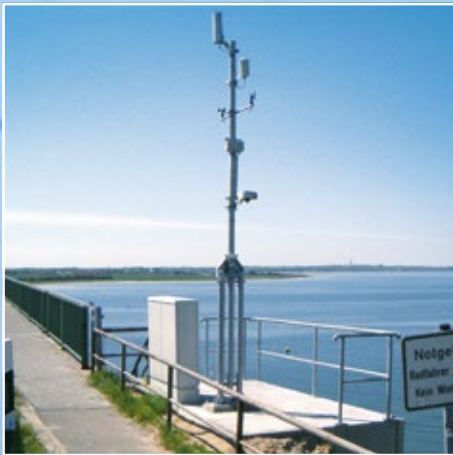
The WS100 is typically mounted on the top of the pole.
